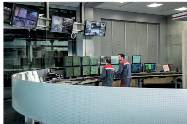
Picture: Control room at Mergelstetten | SCHWENK
